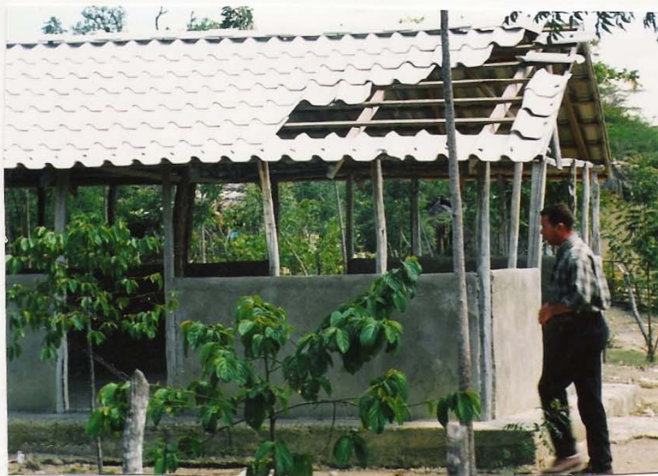
the few tiles which flew away had not been fastened.....
